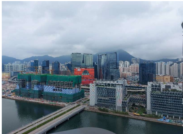
Notable construction activity in Hong Kong at the China Overseas Land development, Kai Tak. Photo Credit: Robert Silgado, Altrinsic Global Advisors
